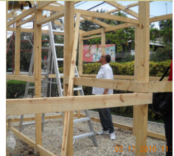
President Moss inspects temporary housing being constructed in Haiti. Dr. Moss spent a week in country in mid-March to get a first hand account of the rebuilding work.
